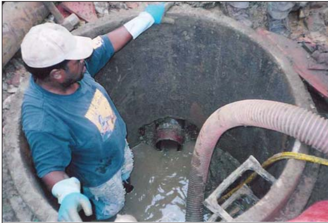
Pictured here is the shallow end manhole that was used as the receiving pit. The new ductile iron pipe can be seen, as it has been pushed into the manhole four to six inches. The cone was removed to facilitate the work for the men.
