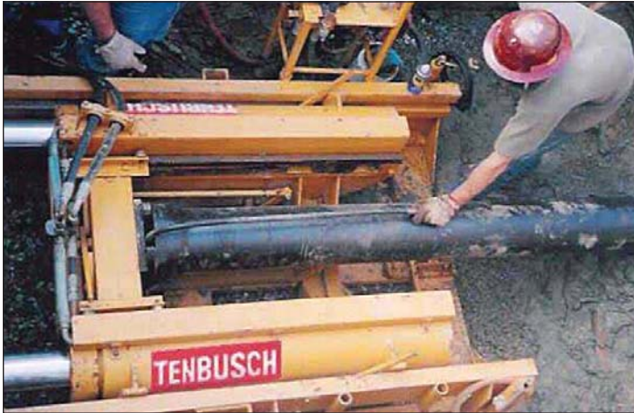
This is the set-up of the Tenbusch Jacking Unit during the Grant Road project.
