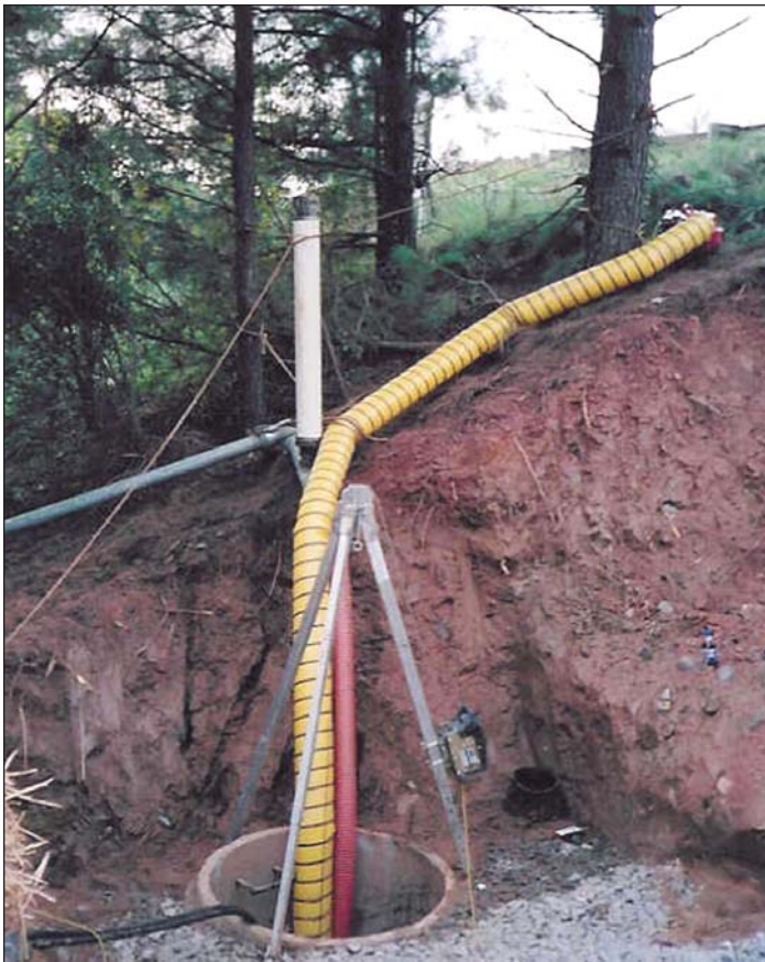
Pictured here is Grant Road and the deep manhole at the north end of the line segment being replaced. By excavating and removing the cone and first section - the manhole depth of 40 feet was reduced to 34 feet.
