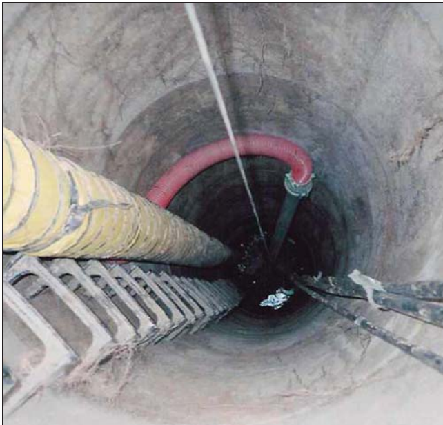
The 34-foot deep manhole served as the receiving pit for the Tenbusch System "lead train." Replacing this manhole would have been especially expensive.
