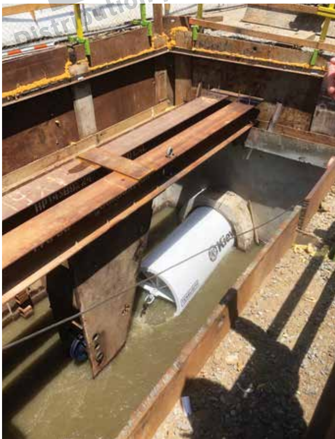
A temporary frame was used to support the cable sheave and pulling cable.
