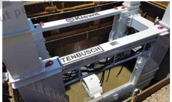
The DD12-150 sliplining jacking unit is shown, ready for the installation of the new pipe.
