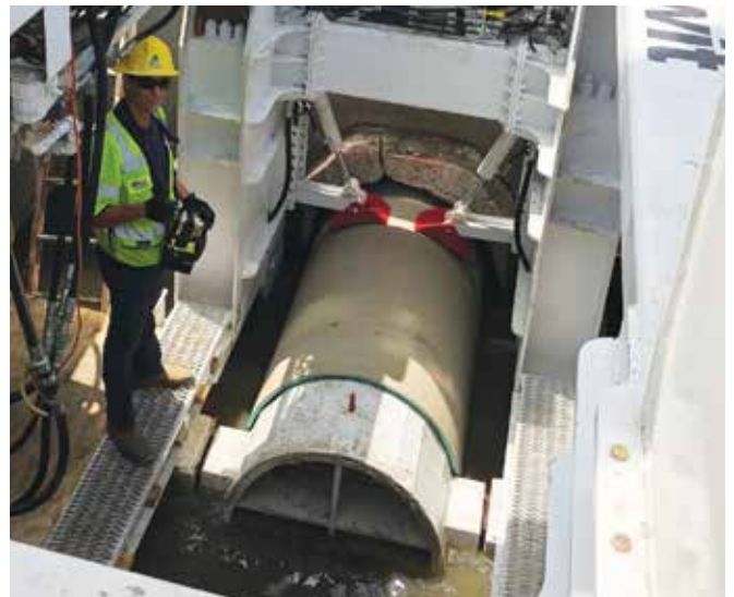
The operator uses a wireless remote-control panel. The photograph also shows the hold-down clamps (in red) used to restrain the previously set pipe while the joint is made up.
