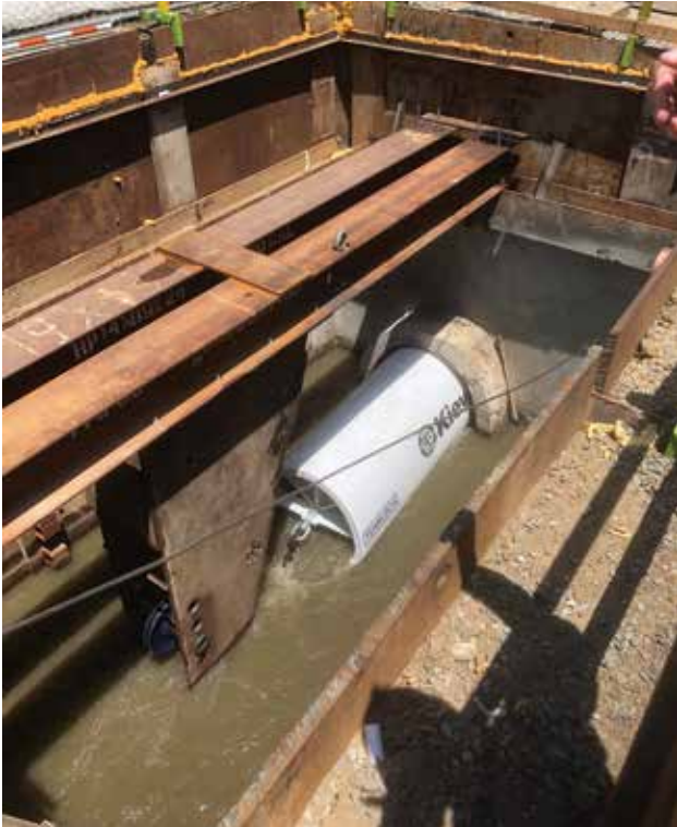
▲ The picture below shows the temporary frame used to support the cable sheave and pulling cable.
