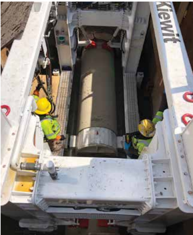
▼ The picture below shows the new pipe being pushed. The machine makes a complete 12' stroke in just one minute and twenty seconds.
