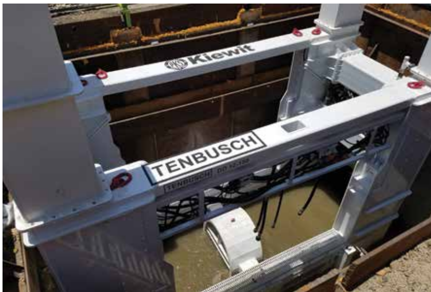
▲ The DD12-150 sliplining jacking unit is shown below, ready for the installation of the new pipe.
