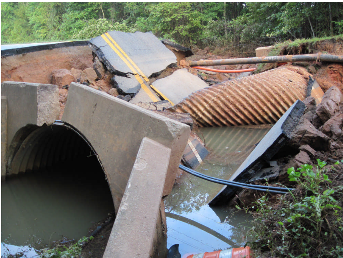
Culvert failures are seldom small and easy to fix. (source for this photo - unknown)
